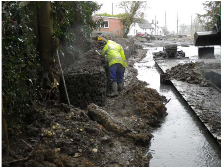
Plate 19. Building of the gabion wall on the south side of the bailey moat, facing west. The ledge is cut into moat infill deposited in the 18th century
