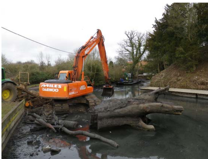
Plate 21. Land-based and barge-mounted excavators clearing the bailey ditch and duck pond viewed from the south
