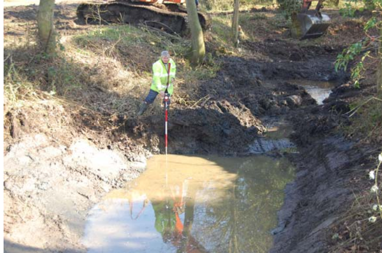
Plate 7. Excavation of the east end of the fishpond (Section 5) during the removal of C20th deposits; brown clay primary silt at the base of the pond has been left in place.
